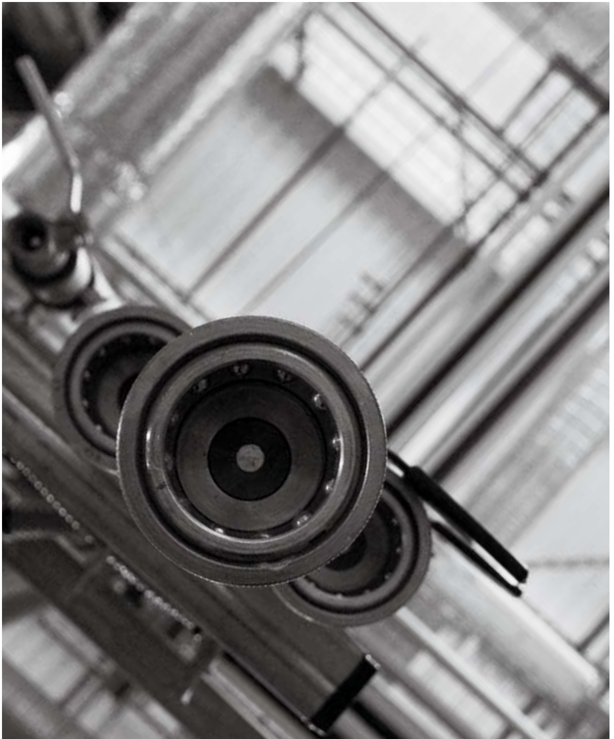
Gas pipes for use at the Repsol Technology Centre located in Mostoles (Spain).
