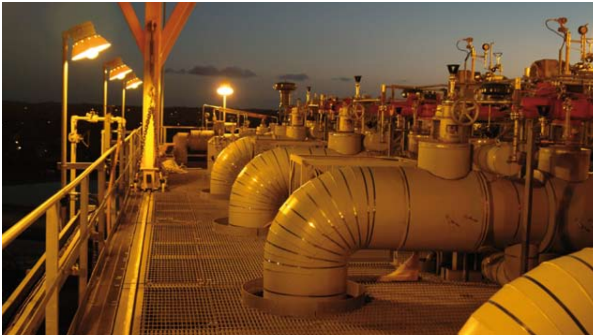
Repsol LNG installations in Trinidad and Tobago.
