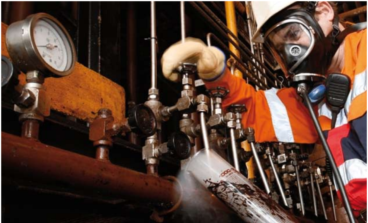
A Repsol operative on Casablanca, the only oil extraction platform in Spain.
