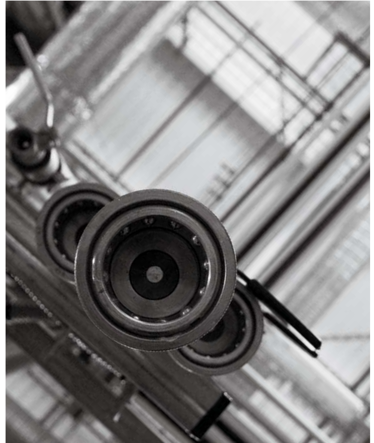
Gas pipes for use at the Repsol Technology Centre located in Mostoles (Spain).
