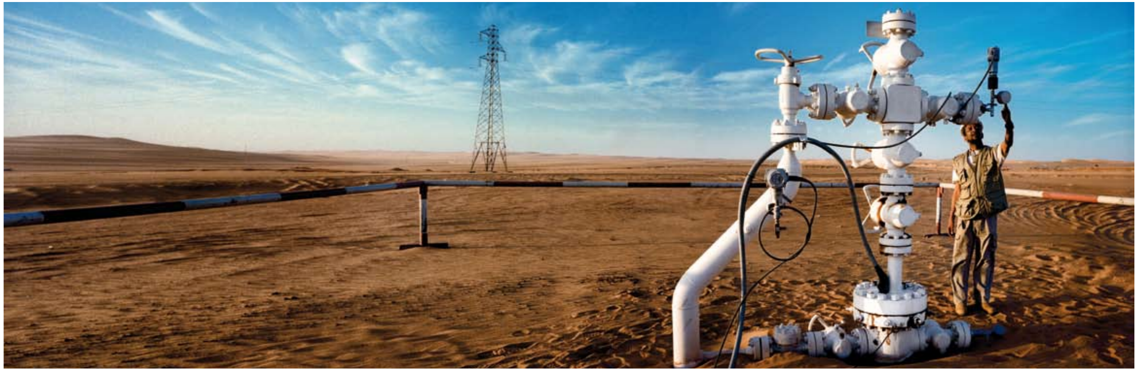
View of a Repsol production field in Libya
