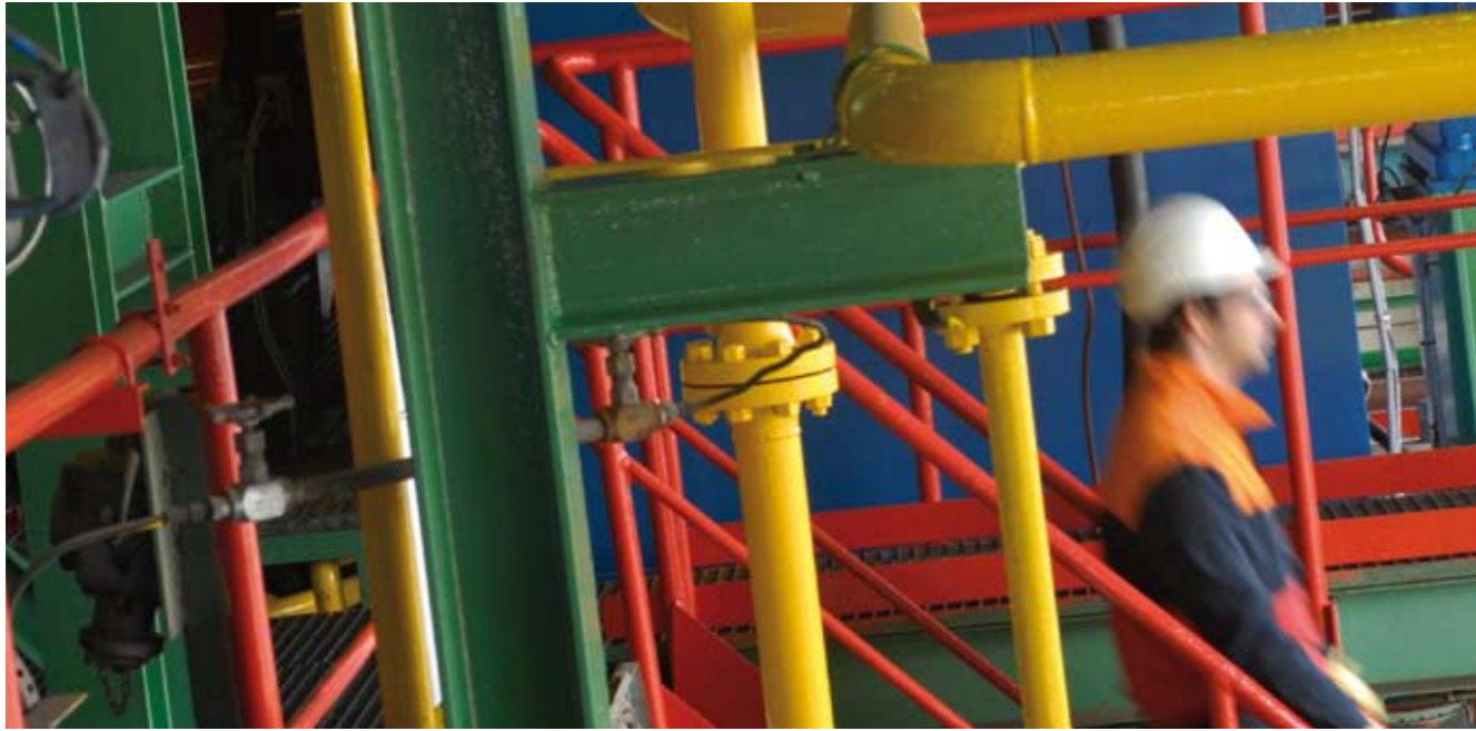
Safety is a priority in all Repsol installations.
