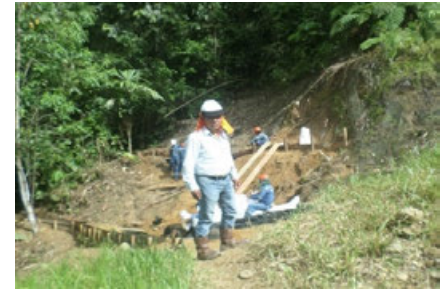
Local monitor in place
